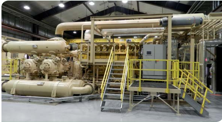
Engine-Compressor Unit, 2370 Horsepower at Cook Inlet Natural Gas Storage Facility; Kenai, Alaska
