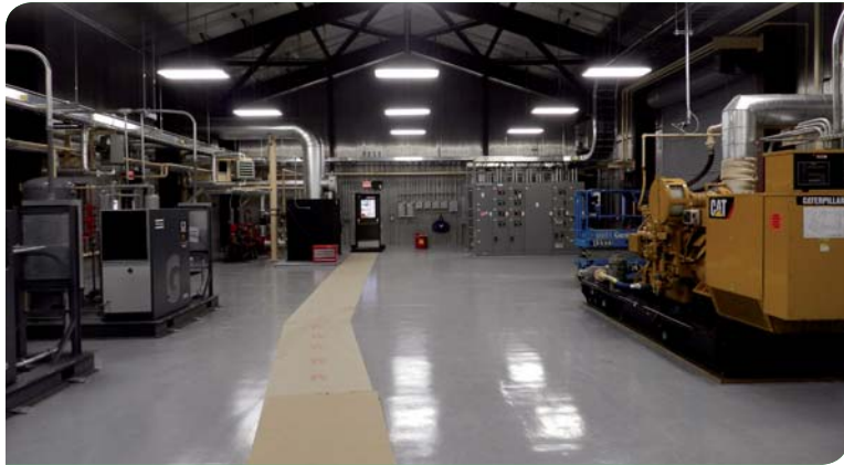
Auxiliary Building at Cook Inlet Natural Gas Storage Facility; Kenai, Alaska
